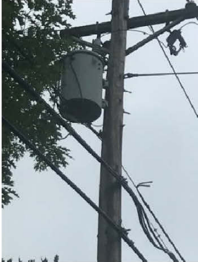
Service Transformer on Depot Road
