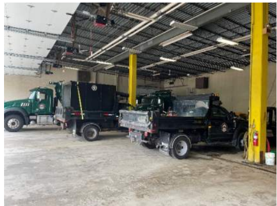
Six Bay Vehicle Storage Garage Propeller Wall Fan Abandoned Hot Water System Covered Propeller Wall Fan
