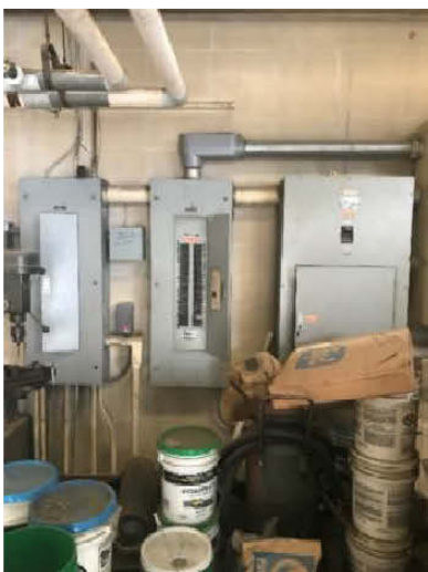
Service Equipment - Six Bay Vehicle Storage Garage
