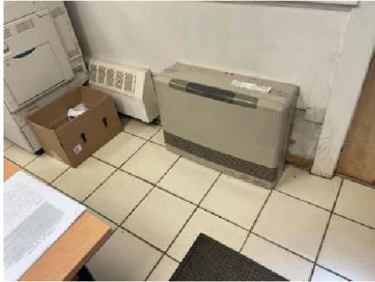
Office Propane Wall Furnace
