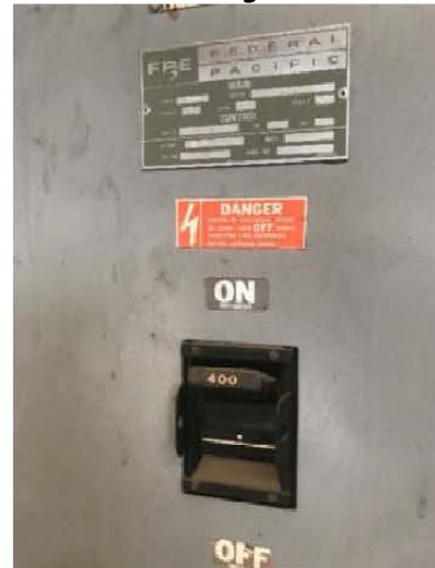
400 Amp, 240 V1, 1-Phase Main Building Disconnect – Mezzanine of Six Bay Vehicle Service Storage Garage
