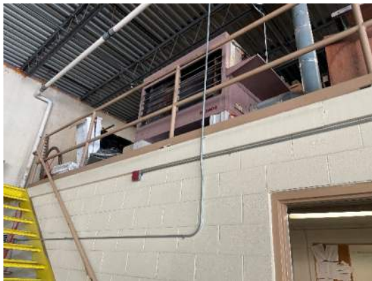
Six Bay Vehicle Storage Waste Heater
