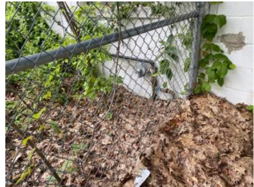
Propane Service Entrance located at the fenced in area adjacent to the Mechanic's Service Garage
