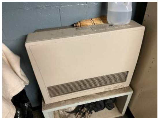
Locker Room/Hall Wall Propane Wall Furnace
