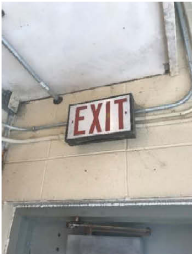
Non-Illuminated Exit Sign - Corridor
