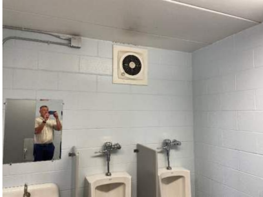
Bathroom Transfer Fan from Breakroom
