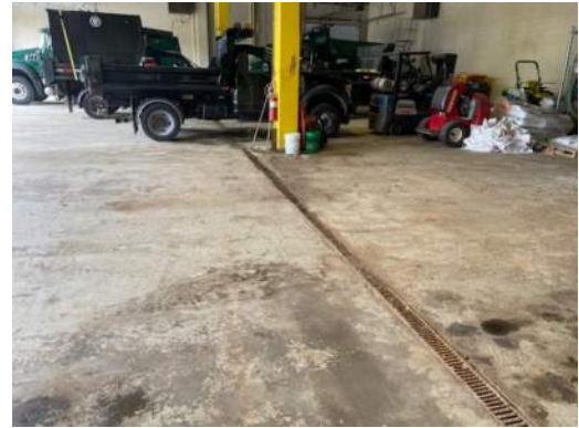
Garage Trench Drain located at the Six Bay Vehicle Storage Garage
