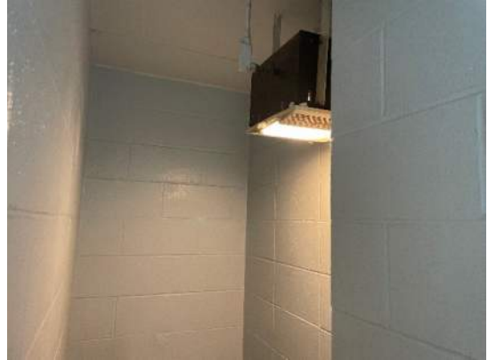
Bathroom Ceiling Exhaust Fan
