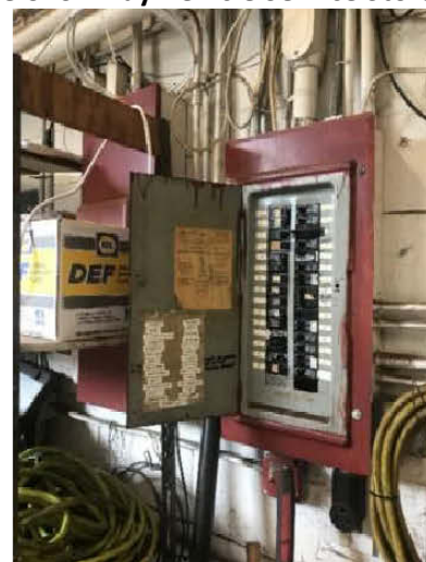
Panelboards – Mechanic's Service Garage
