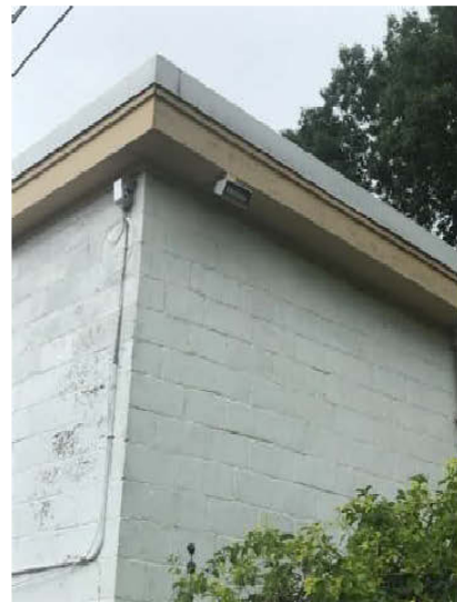
Exterior Wall Pack – Office Building
