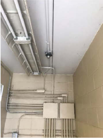
Industrial Fixture/Heat Detector – Six Bay Vehicle Storage Garage
