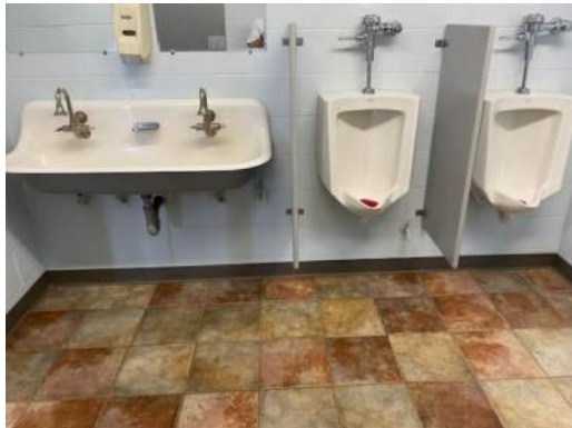
Plumbing Fixtures at the multi user Men's bathroom
