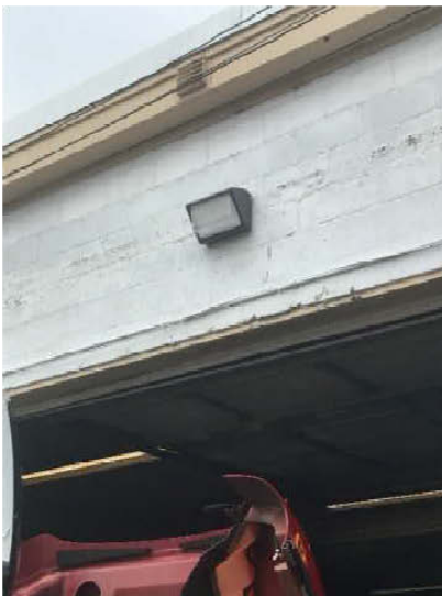
Exterior Wall Pack - Six Bay Vehicle Storage Garage
