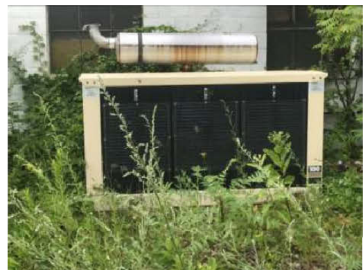
100 KW, 120/240V 1-Phase Generator – Exterior Fenced -In Area
