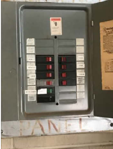
Panelboards – Mechanic’s Service Garage
