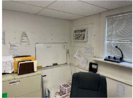
Office Through Wall Air Conditioner
