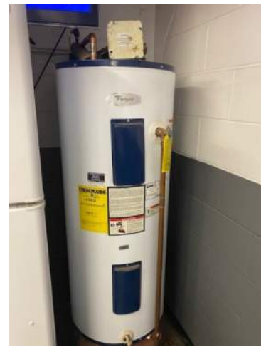
Electric Hot Water Heater at the Breakroom
