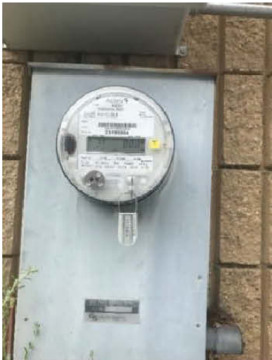
Electric Meter – Six Bay Vehicle Storage Garage
