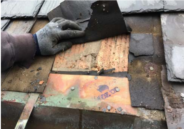
Photo 8: The slate, underlayment, and copper gutter are nailed directly into the terra cotta roof deck.
