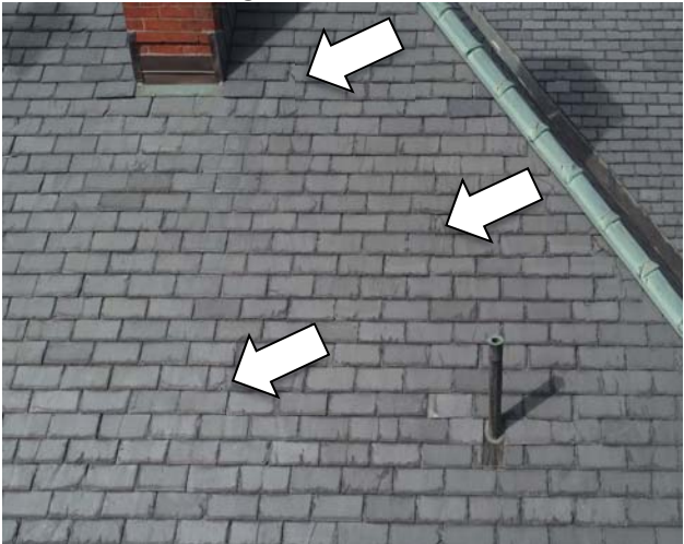
Photo 16: View of typical broken shingles.
