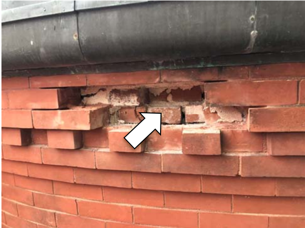
Photo 7: View of test cut 1 at the masonry directly below the gutter. Note the cracked brick and deteriorated mortar in the second wythe of brick.
