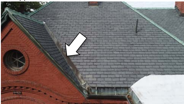
Photo 23: View of deteriorated sheet metal valley flashing.
