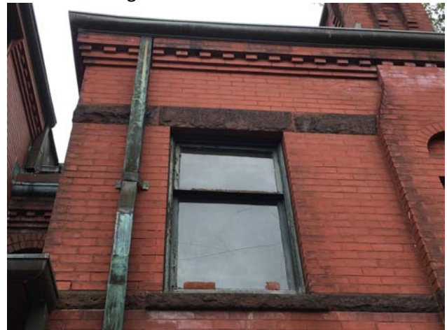
Photo 34: View of cracked glazing and loose brick masonry units on the brownstone sill.
