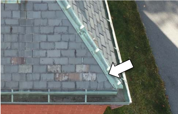
Photo 17: View of a loose slate.
