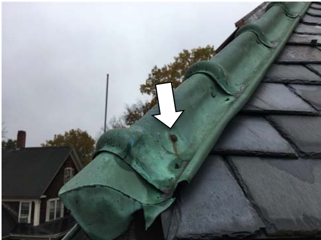
Photo 28: Sheet metal fasteners appear rusted in some locations.
