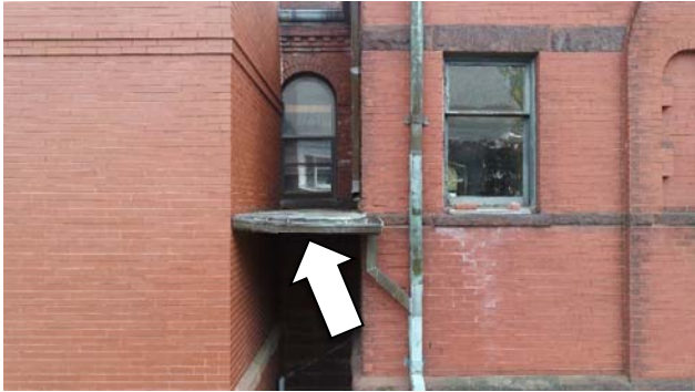
Photo 26: View of a deformed gutter.
