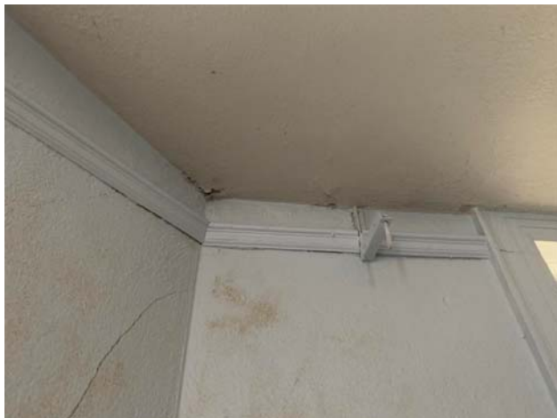
Photo 2: View of peeling paint, cracked plaster, and water staining on the basement floor walls at Leak Location #1.
