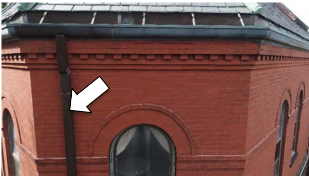
Photo 22: View of a downspout resting against the face of a wall.
