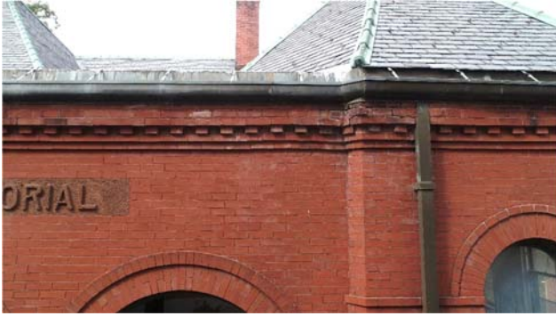
Photo 31: View of the deteriorated mortar and white colored efflorescence staining.
