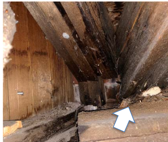
Photo 4: View of rotted wood at the end of the roof framing valley beam Leak Location #4.
