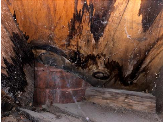
Photo 5: View of water staining on the underside of the roof sheathing at Leak Location #4.
