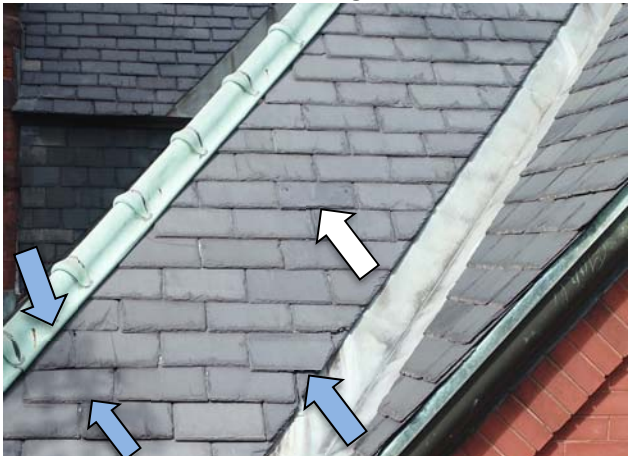
Photo 19: View of exposed slate fastener holes. Note also the loose slates (dark arrows).
