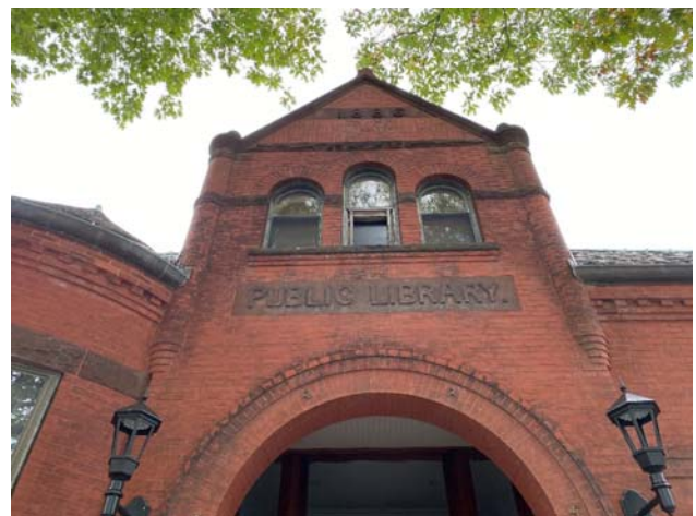
Photo 35: View of missing glazing.
