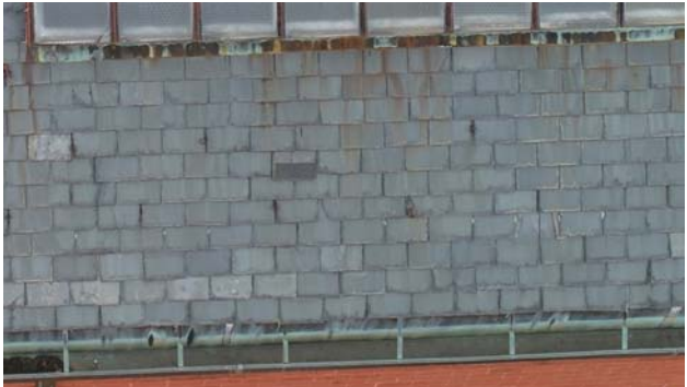
Photo 18: View of a missing shingle.
