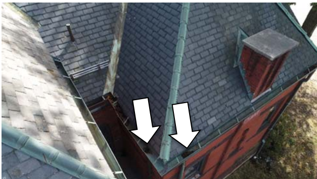
Photo 27: View of two obstructed downspouts.
