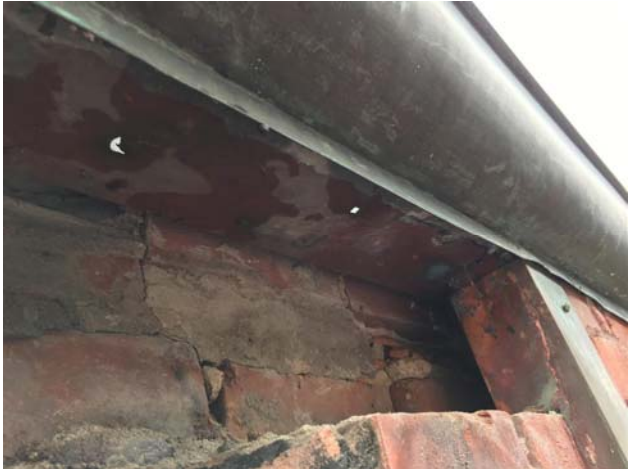
Photo 9: View of punctures in the gutter at test cut 2.
