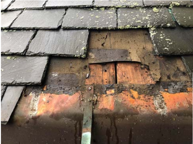
Photo 6: View of test cut 1 at the roof with a wood roof deck.
