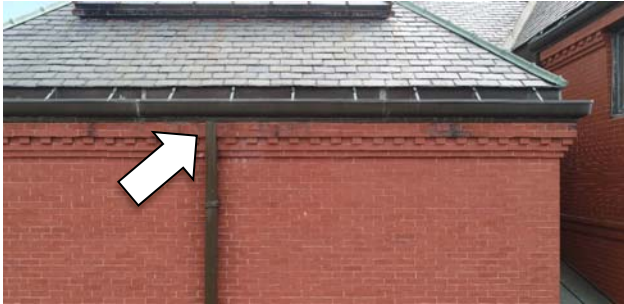
Photo 21: View of a downspout integrated into the top courses of masonry at a wall.
