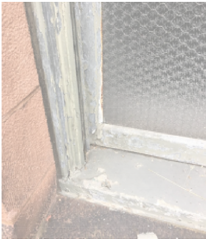
Photo 37: View of a window with peeling paint.
