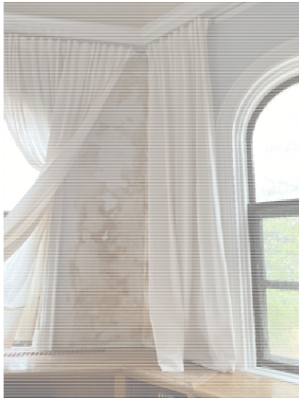
Photo 1: View of heavy water staining on the first floor walls at Leak Location #1.
