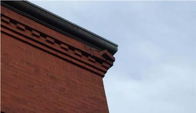
Photo 30: View of the displaced brick in danger of falling.
