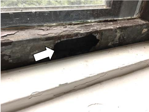
Photo 36: View of window with a rusted hole in the frame.
