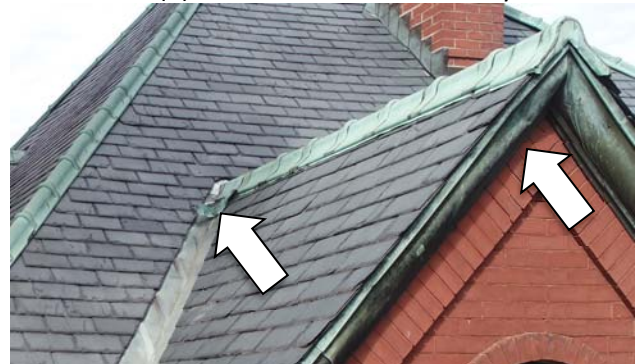
Photo 25: View of deformed and displaced ridge cap and rake trim.
