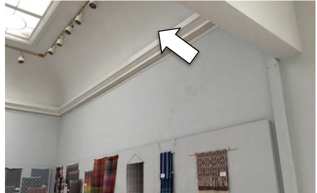
Photo 3: View of Leak Location #2.
