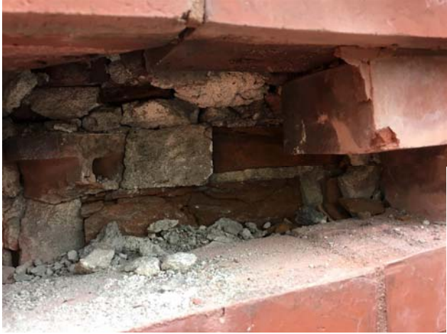
Photo 10: View of cracked brick and deteriorated mortar in the second wythe of masonry.
