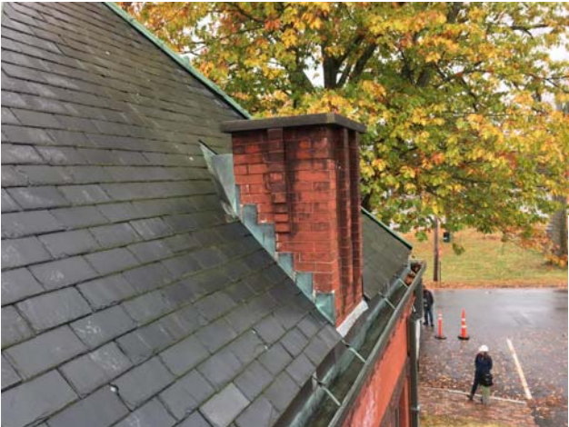
Photo 29: The sealant along the sheet metal flashing is failed, and the brick masonry appears stained at this chimney.
