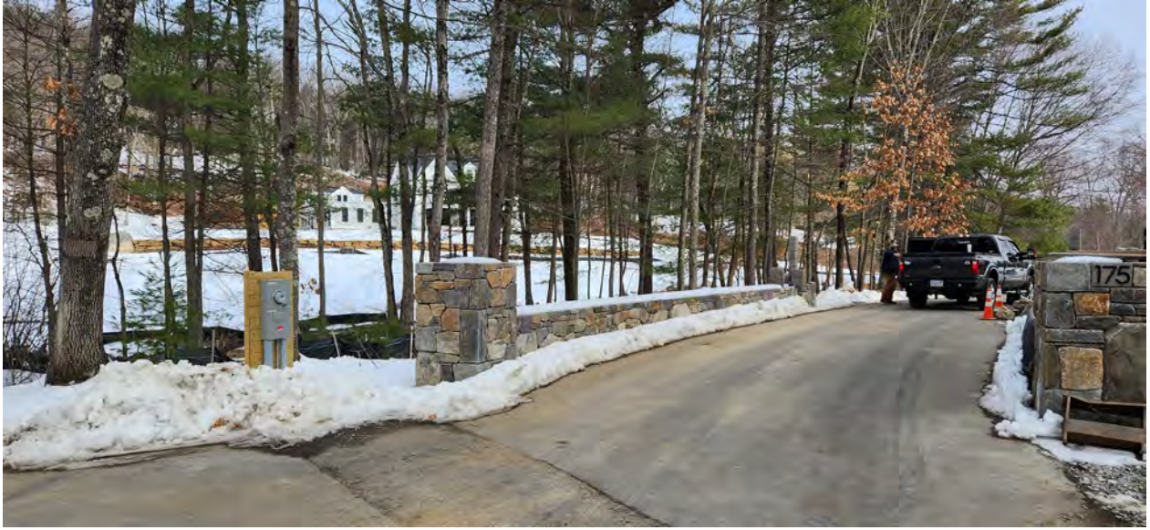
[Site Photo 1 – Stonewalls prior to relocation. See elec. meter for point of reference]
