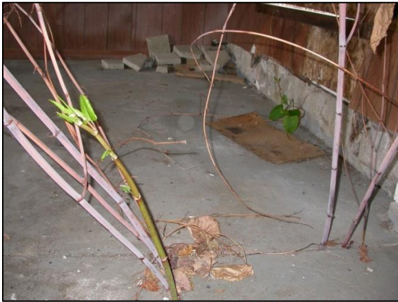
Structural damage to residential home/basement
