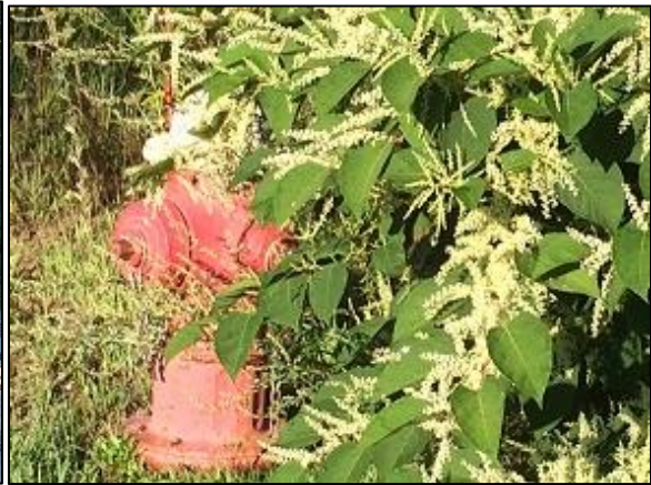
Obstruction of fire hydrant
