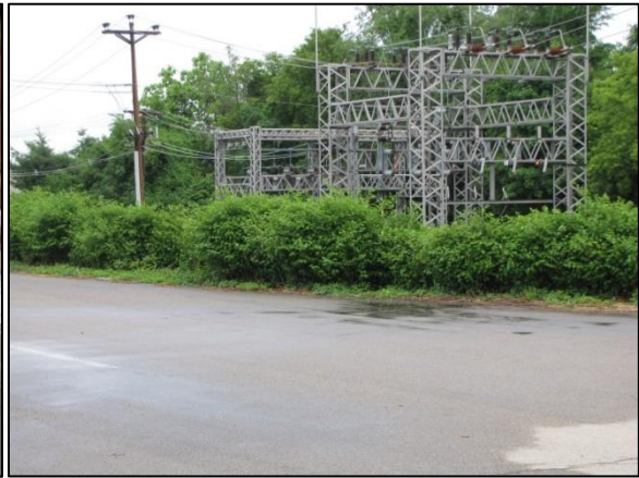
Power grid sub-station impacts
